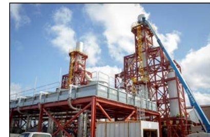
Schofield Barracks, HI: Lease Project: 50 MW / 30 day contingency microgrid where Hawaiian Electric constructed, owns, operates and maintains a 50 MW multi-fuel power generation plant, fuel storage tanks, and controls.
