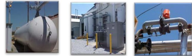
Anniston Army Depot, AL: UESC Replacement and Modernization of Depot-wide central heating and process high pressure steam plants, HVAC equipment and controls, interior and exterior lighting, compressed air equipment and distributions, and potable water fixtures.
