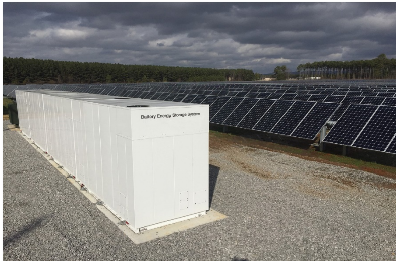
Army's First Privately Funded, Economically Viable Battery Storage System
